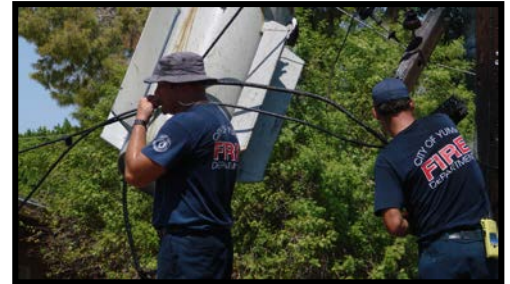
City of Yuma Fire Fighters remove downed electrical wires following a seasonal wind storm.
